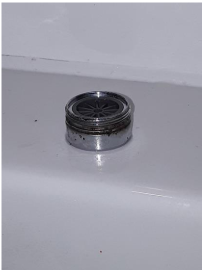
Tap Diffuser Condition
