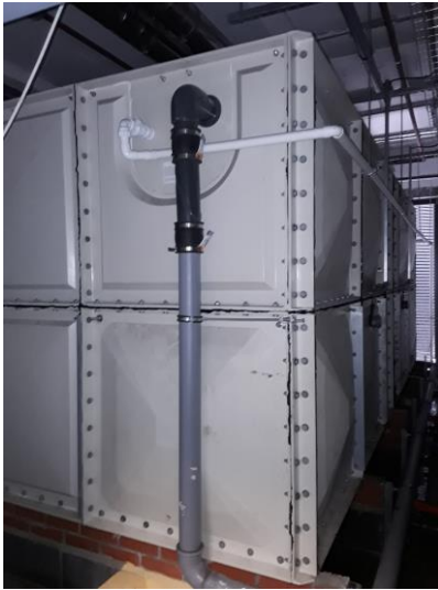
Screened Overflow Pipework
