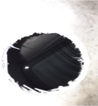
Missing lid vent causing potential contamination risk
