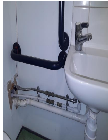
Dead Legs at Toilets – 2-017
