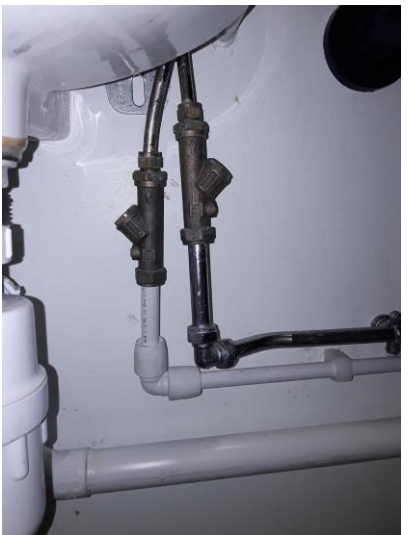
Example of Y-strainers at Mixer Taps
