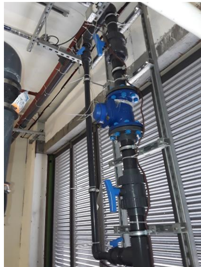
Bypass on Mains Water Pipework
