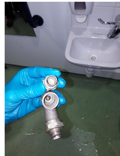
Example of Y-strainer Condition
