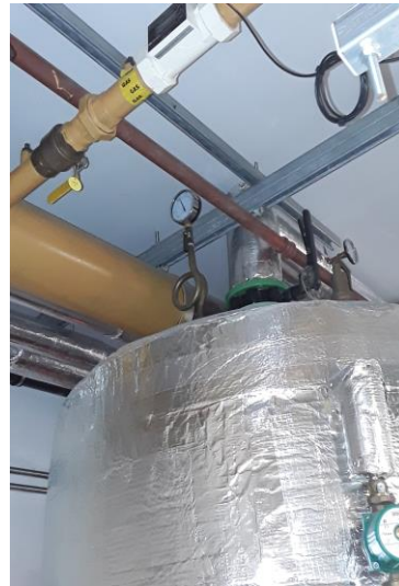
Pigtail Pipework to Gauges
