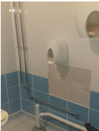
Possible Dead Leg Pipework in Hydrotherapy Room
