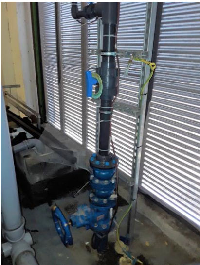
Incoming Mains Water Pipework
