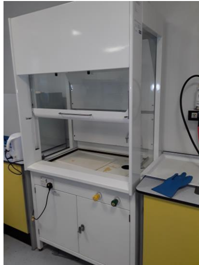
Example of Lab Fume Cabinet Ensure Regular Use
