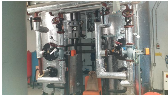
Boiler Room Calorifiers 1 & 2
