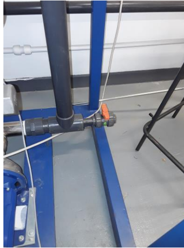
Booster Pump Drain Line
