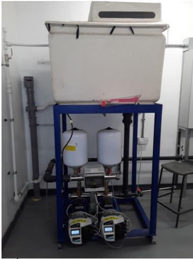
2 nd Floor Lab Tank
