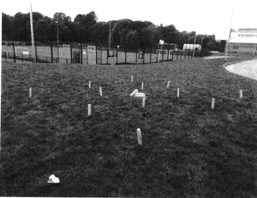
Setting out of stakes to mark HP10 delineation locations prior to remedial works
